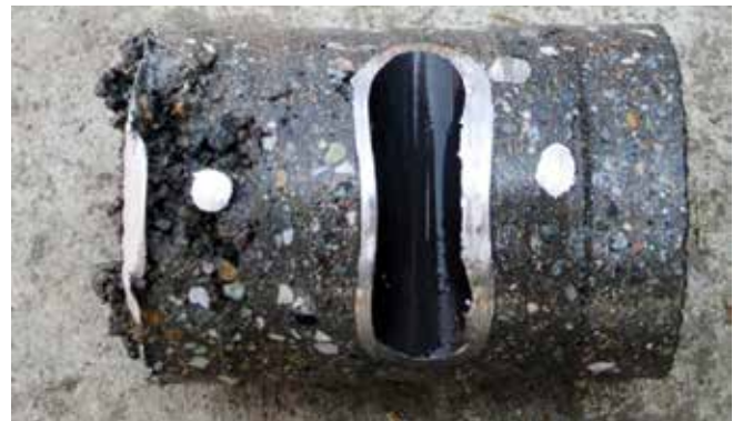
Fig. 11: Side view of Core No. 1. Note voids around back layer of reinforcing bar near stay-in-place form. Assigned ACI Core Grading No. 4
