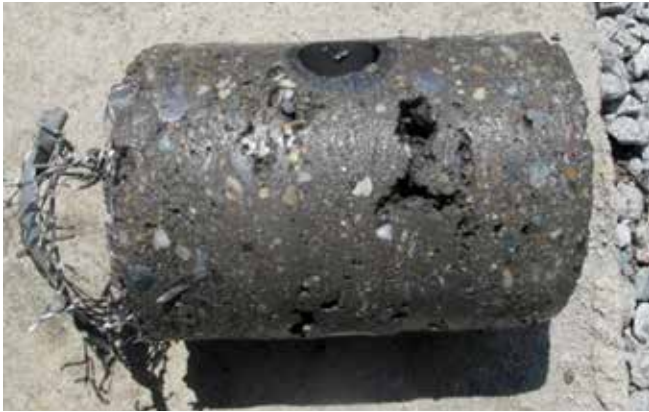
Fig. 13: Side view of Core No. 3. Note voids in front of cooling pipes. Assigned ACI Core Grade No. 3
