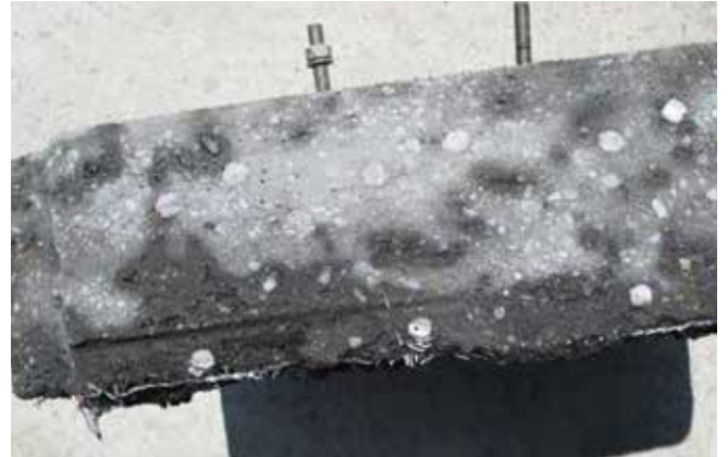
Fig. 10: View of top of slab removed from high wall. Note voids behind cooling pipe and back reinforcing bar
