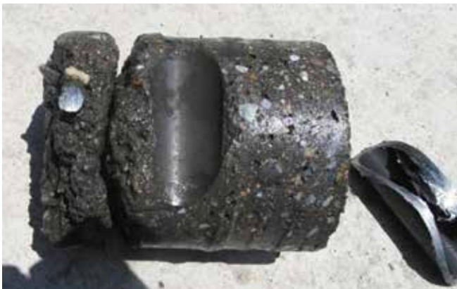
Fig. 15: Side view of Core No. 5. Core broke in two at porous zone behind cooling pipe. Assigned Core Grade No. 4
