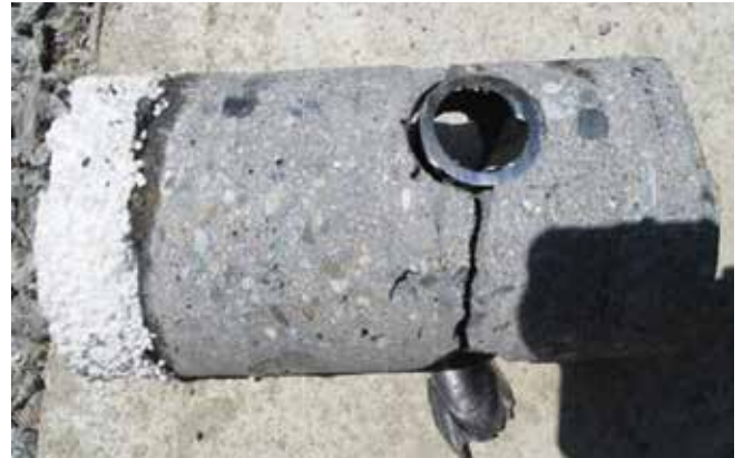
Fig. 16: Side view of Core No. 6 from invert. Shotcrete well consolidated and assigned ACI Core Grade No. 1
