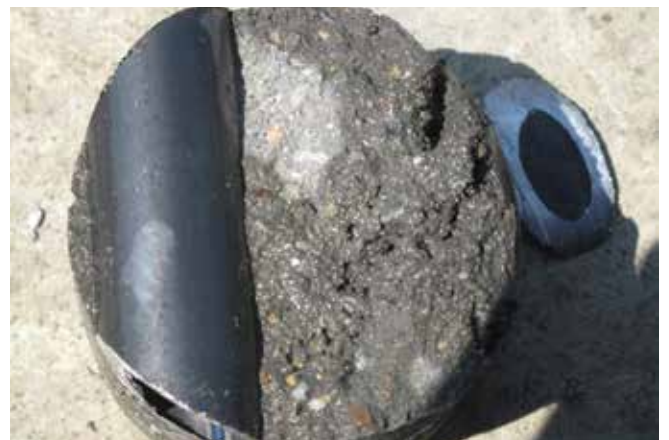
Fig. 12: View of middle of Core No. 2. Note porosity behind cooling pipe. Assigned ACI Core Grade No. 3
