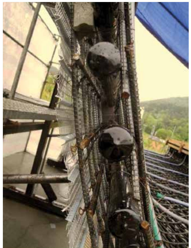
Fig. 2: End view of reinforcing steel, cooling pipes, and Stay-Form in high wall
