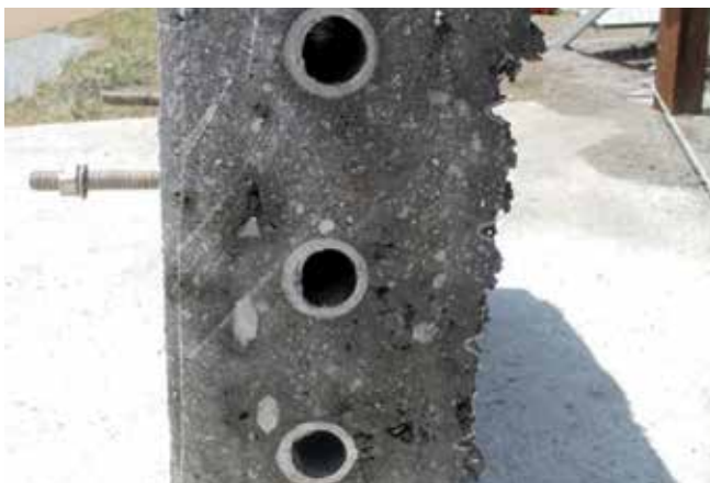
Fig. 9: View of right side of slab removed from high wall. Note typically good encapsulation of reinforcing bar and cooling pipes
