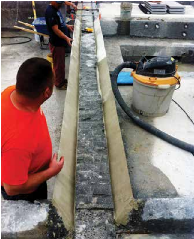
Fig. 3: Construction included the special slot-drainage system built into the narrow wall dividing the pool and spa
