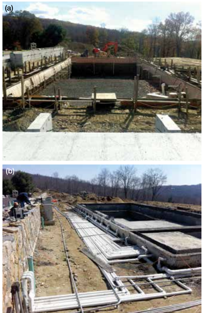
Fig. 2(a) and (b): The pool and spa cover a lot of ground—nearly the size of a regulation tennis court, which meant using a massive amount of reinforcing steel and pipe, and keeping track of the large number of PVC lines as they moved toward and into the equipment vault/surge tank bunker
