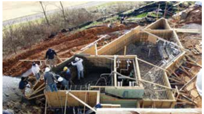
Fig. 1: Rigid and easily removable forms allow for sturdy steel work and shotcrete placement while being able to strip the forms and shoot the other side
