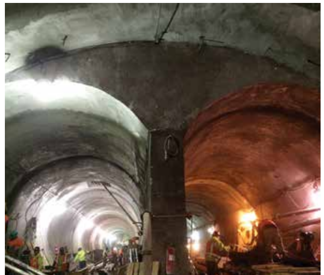
Fig. 5: Complete CM006 M-Cavern arches, end wall tunnels, and center walls showing rubber float finish
