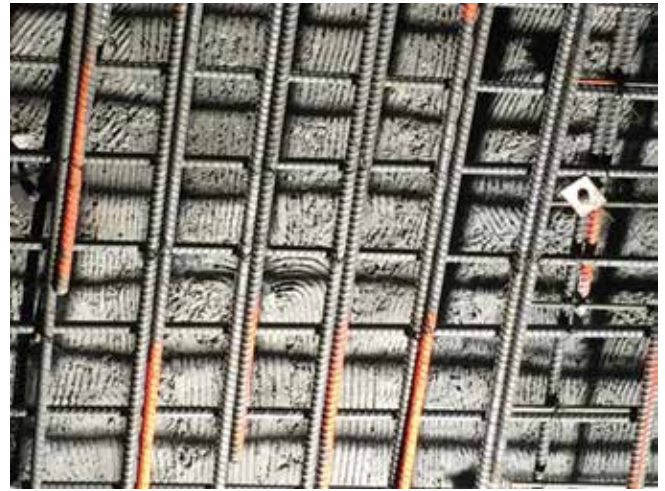
Fig. 4: First layer of shotcrete at CM006 showing scratch finish prior to installation of inside face reinforcing bar
