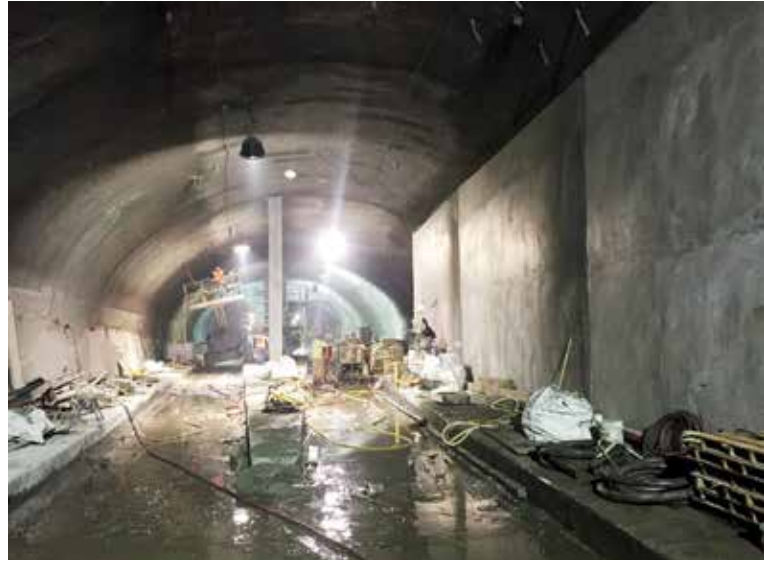
Fig. 13: Finished Grand Central Terminal 1/2 arch with rod finish; walls were rubber float finish
