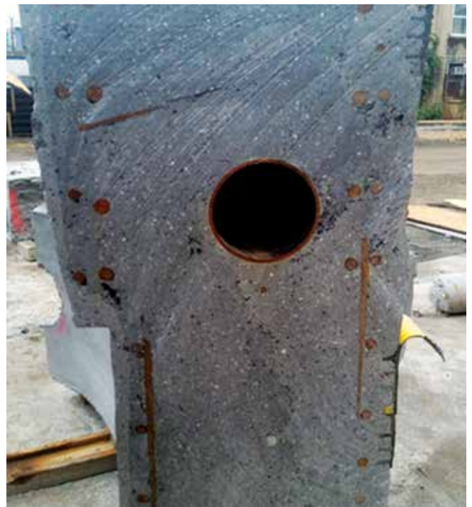
Fig. 7: Encapsulation around reinforcement, embedments, and encasement of water barrier (on right lower side)
