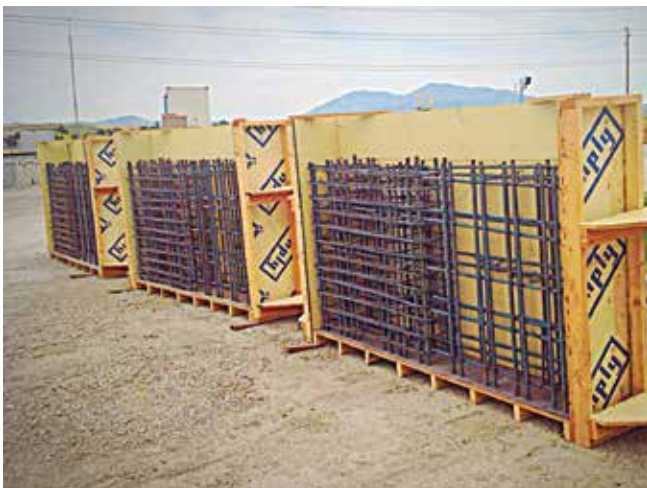
Fig. 1: Mockup panels with congested reinforcement patterns may require alternative methods to attain adequate consolidation
