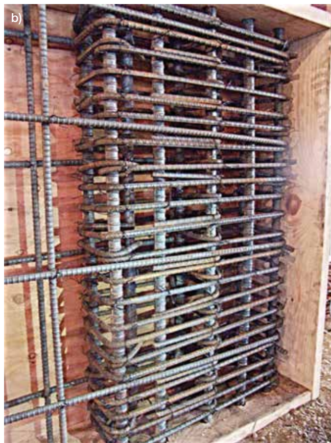
Fig. 2(a) and (b): Mockup panels with congested to extremely congested reinforcement patterns
