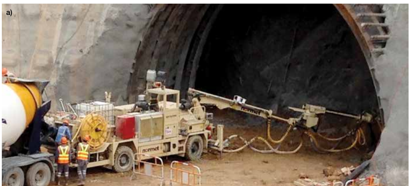
Fig. 1: Sprayers in action: (a) tunnel portal spraying with Spraymec 8100 VC; (b) equipment suitable for small, medium, and large headings; and (c) delivery and shotcrete application in mining projects around the world
