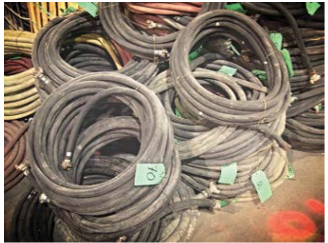
Fig. 3: Larger-diameter air supply lines may be necessary to maintain sufficient nozzle velocity
