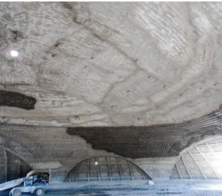
Fig. 1: Reinforcing bars and shotcrete are integral parts of the dome construction process
