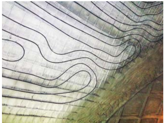
Fig. 4: An innovative system of piping runs throughout the shotcrete
