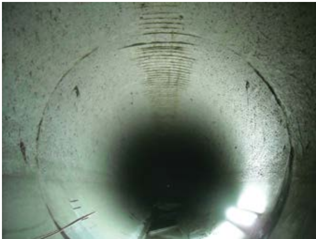
Fig. 1: Initial conditions—note deterioration at the top of the drainage tunnel
