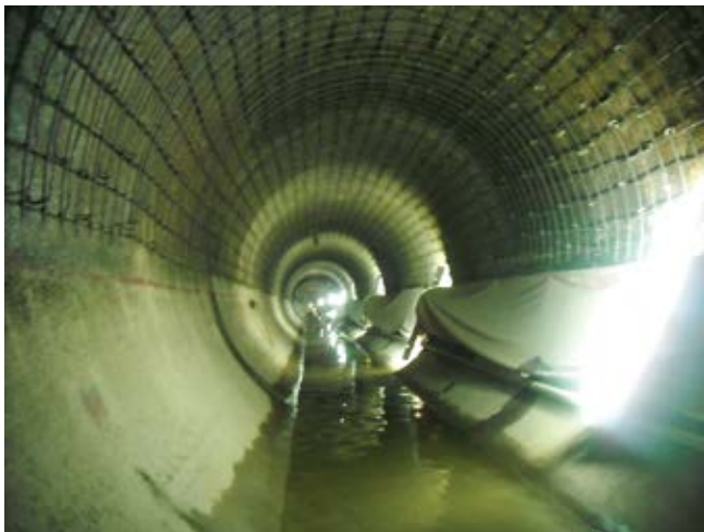
Fig. 2: Surface prepared and supplemental reinforcement in place ready to cover with shotcrete
