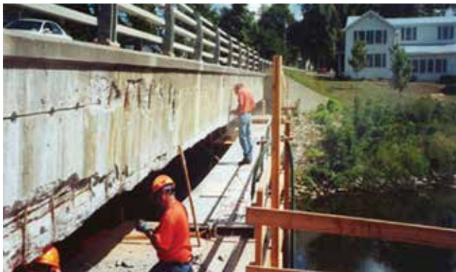
Fig.3: Type 2 anodes are placed in series into drilled in holes in the existing concrete prior to shotcrete application
