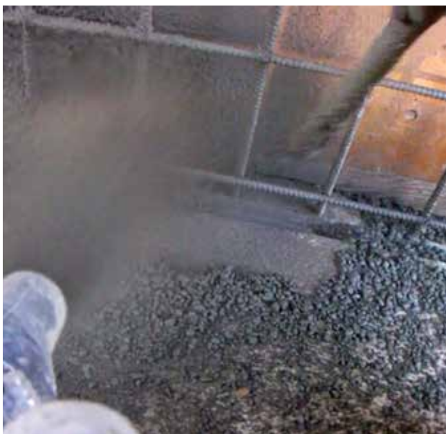
Fig. 4—Blow pipe operator continuously maintains a clean receiving surface by working ahead of nozzle stream
