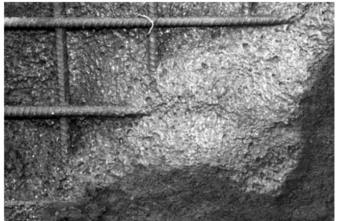
Fig. 2(a)—This freshly applied surface glistening with paste is evidence that the slump is ideal. Reinforcement bars are clean, without buildup. Fast-moving aggregates within the nozzle stream have become deeply embedded within the shotcrete surface, leaving a smooth, shiny paste layer
