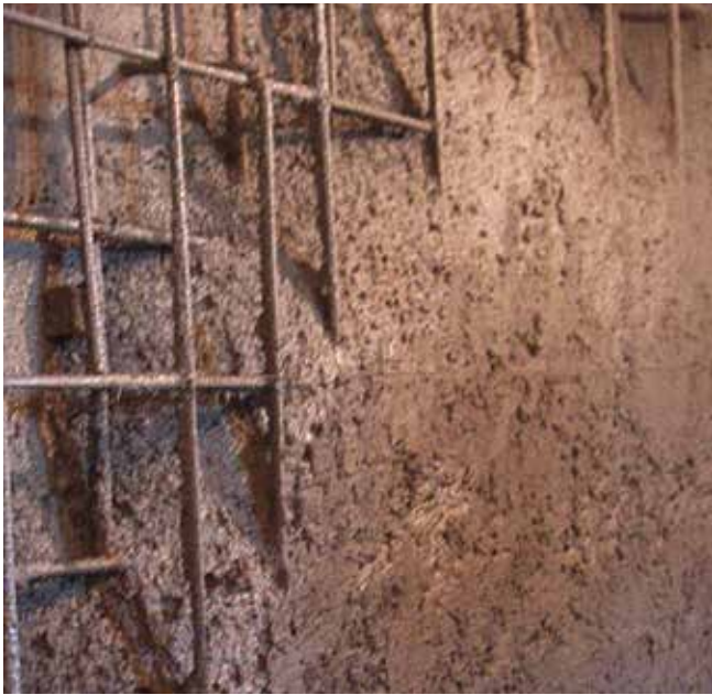
Fig. 5(a)—Maintain a relatively sharp angle and completely cover reinforcements to encourage rebound to fall free of the work
