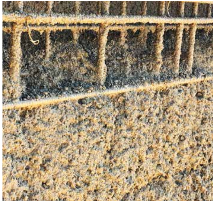
Fig. 5(b)—Close-up reveals what can occur when reinforcement is not properly covered by the nozzleman. Rebound will become trapped by the deposition of additional material if it is not blown free of the work. This is the likely cause of the flaws within the test specimen in Fig. 1
