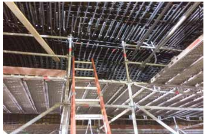
Fig. 4: Tunnel and cross-passage intersection arch reinforcing bar upper-level arch of TT#1 structure
