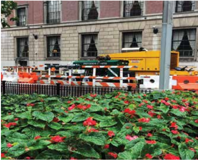
Fig. 13: Pump location at intersection of 37th and Park in New York, NY, for the placements in upper-level arch of TT#1 structure
