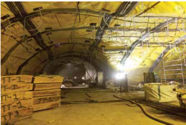
Fig. 2: Waterproofing membrane installed after build back and smoothing has been completed in the upper-level arch of TT#1 structure
