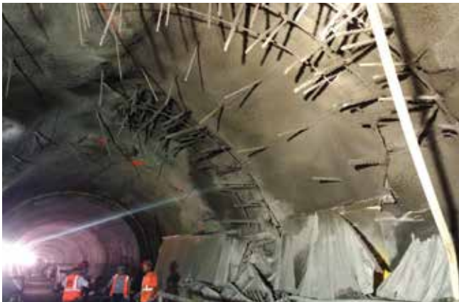
Fig. 1: Upper-level arch section of three-level structure TT#1. Overbreak reinforcement dowels and grade control wires
