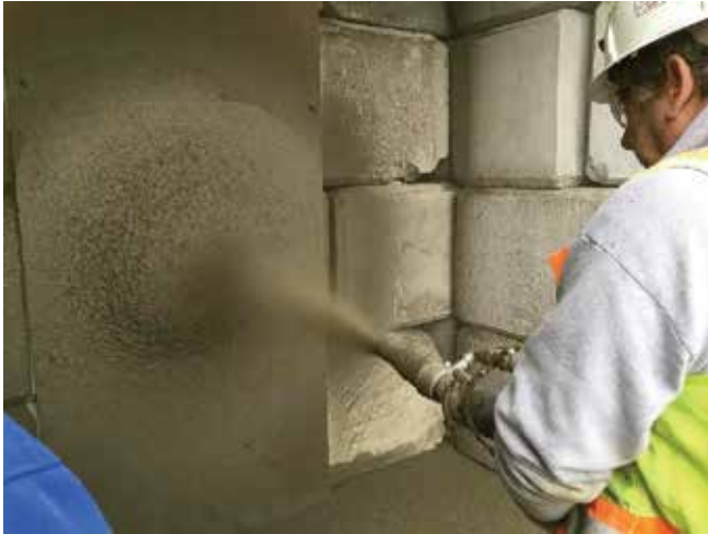
Fig. 5: Shooting a beehive of plain concrete mixture (WP) 6 in. (150 mm) thick on a vertical plywood panel
