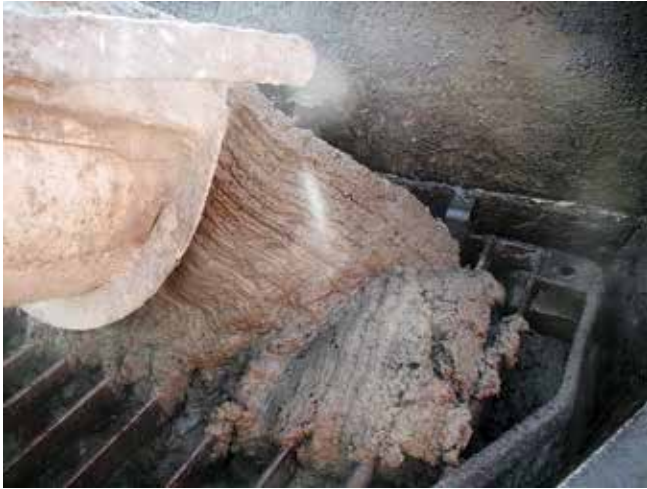
Fig. 12: Natural fiber-reinforced shotcrete (Mixture B) being discharged from concrete truck chute into pump hopper; note highly cohesive nature of mixture
