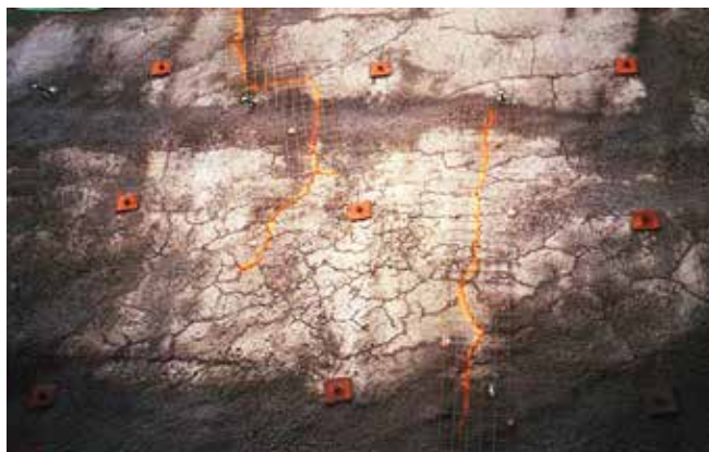
Fig. 1: Plastic shrinkage cracking in shotcrete slope stabilization
