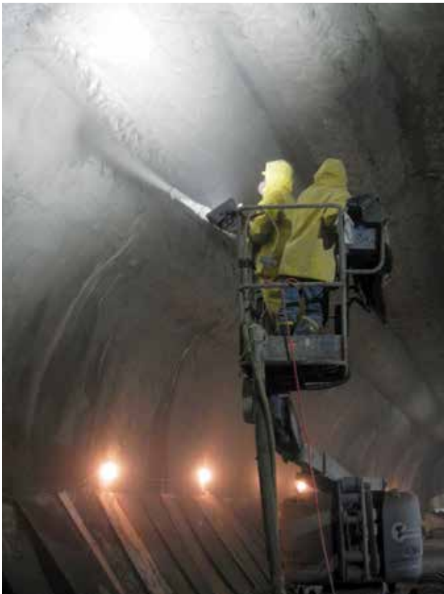
Fig. 7: Adequate lighting and access to the shooting face in a tunneling application (from Crouch, 2014)
