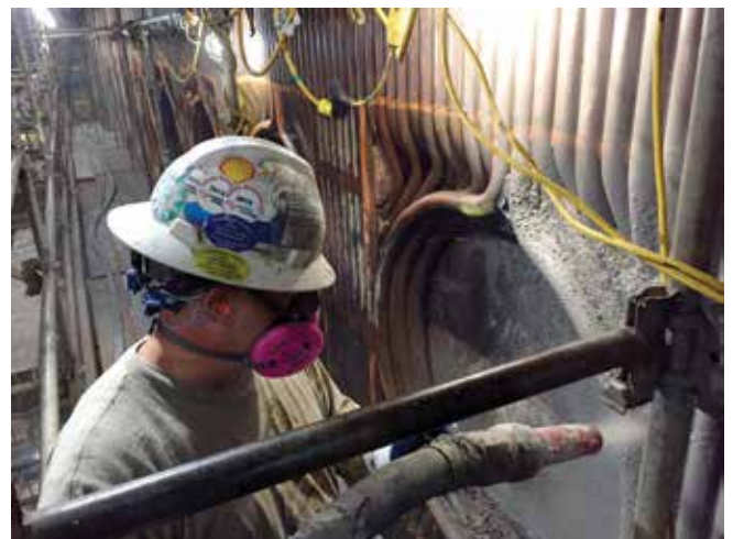
Gunning a high-temperature refractory with the dry-mix process in the burners of a coal-fired power plant. The refractory material did not use portland cement
