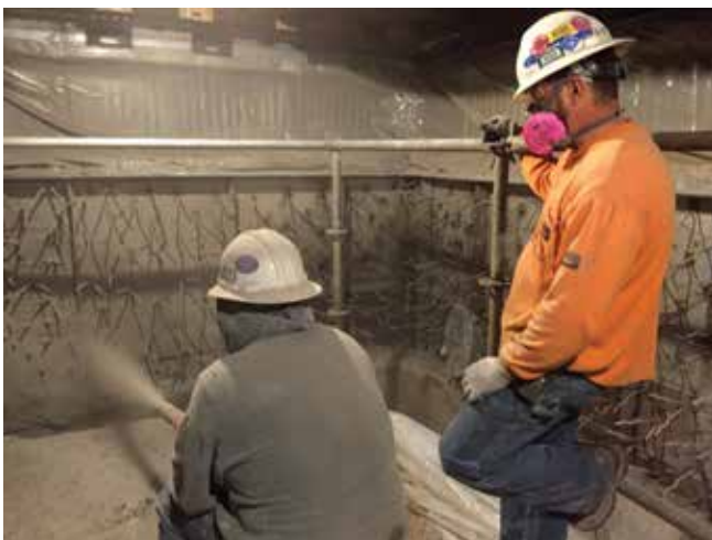
A 9 in. (225 mm) thick dry-mix process installation of high-strength 2600°F (1400°C) refractory in a power plant ash hopper
