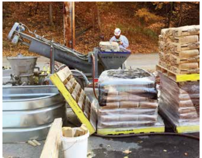
A typical setup used in dry-mix process refractory installations with a rotary gun and an auger-type pre-dampener for gunning dry prepackaged refractory material
