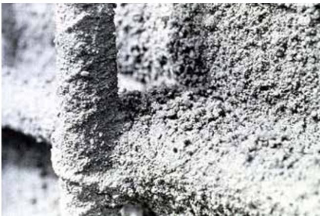
Fig. 2: Visual observation during shotcrete observation may note improper shooting techniques, resulting in inclusion of voids or rebound materials with low integrity where it matters most. Laboratory tests of panel cores do not address this issue, as it is related to shooting technique in this location. Visual examination for cracking patterns, supplemented by hammer sounding (ASTM C4580-12) to detect hollow/delaminated areas for closer study, and possible coring for laboratory testing where relevant properties can be determined
