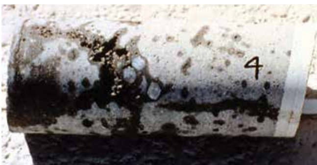
Fig. 3: Visual inspection of cores extracted from structures with unusual cracking or leaking can help to reveal improper shooting techniques or poor materials. All concrete has some degree of void or less than perfectly consolidated materials. Using an ACI Certified Nozzleman and crew that works well together to avoid inclusion of rebound is critical
