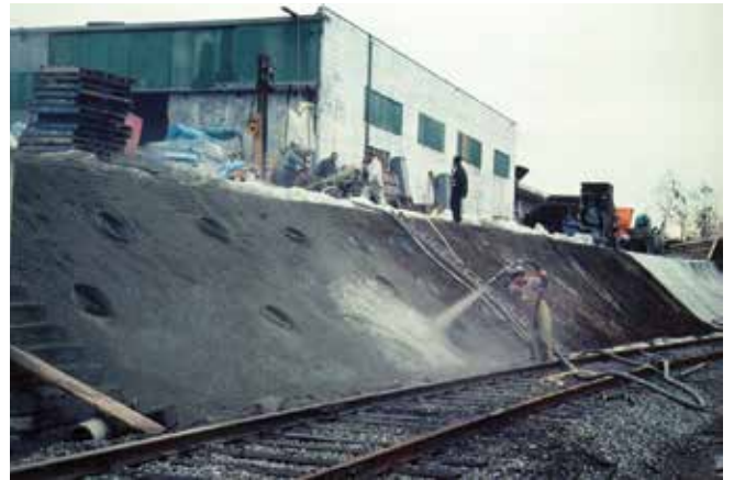
Fig. 4: Dry-mix steel FRS lining of a railway embankment in Burnaby, BC, Canada, in 1978
