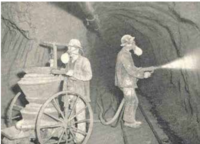
Fig. 2: Lining a tunnel with gunite using a double-chamber gun in the 1920s
