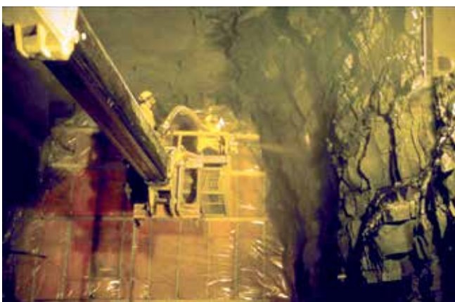
Fig. 6: Hand application of dry-mix shotcrete in a tunnel in British Columbia, Canada, in the 1970s
