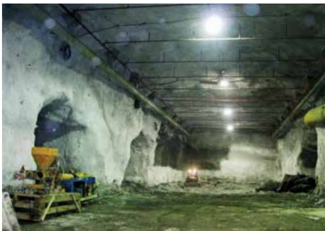
Fig. 9: Large underground opening for workshop in mine in Sudbury, ON, Canada, lined with macrosynthetic FRS
