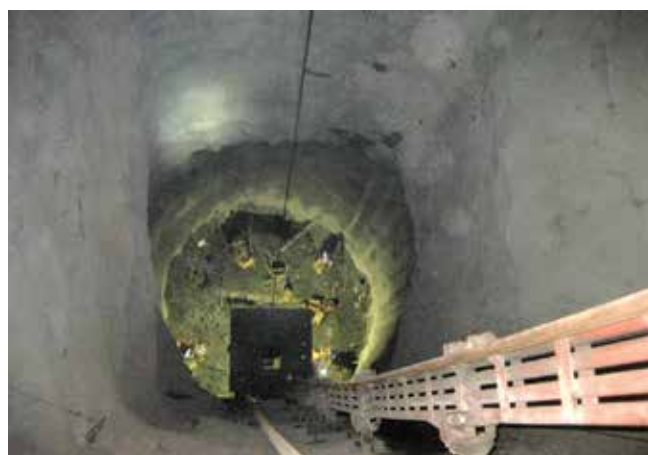
Fig. 3: Construction and installation of protective shotcrete lining for critical ore pass in a Northern Quebec gold mine
