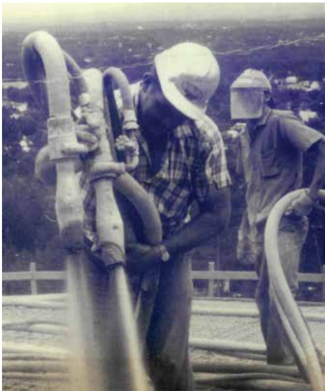
Fig. 2: Placing dry-mix shotcrete using dual nozzles to increase production when shooting a free span 3 in. (76 mm) thick dome circa 1965
