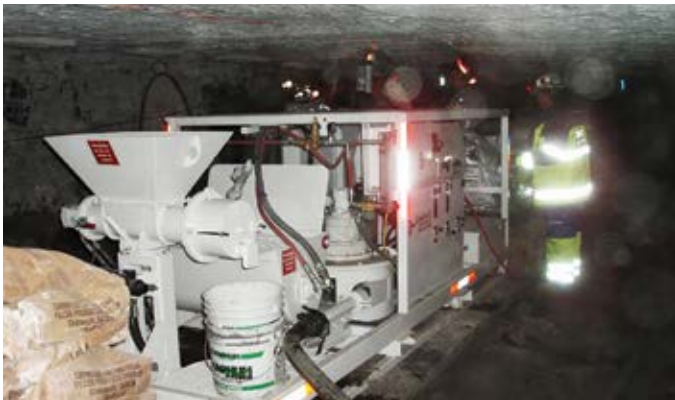
Fig. 3: Squeeze pump underground
