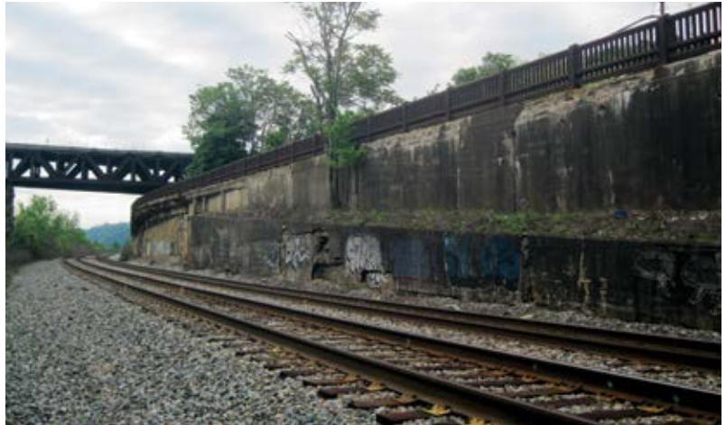
Fig. 2: In many cases, the shotcrete repair areas are close to the railroad tracks and special precautions have to be taken on active lines
