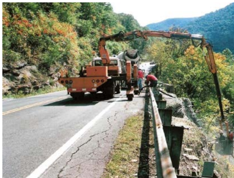
Fig. 1: A Snooper inspection crane being used for hillside access above railroad line during shotcrete placement
