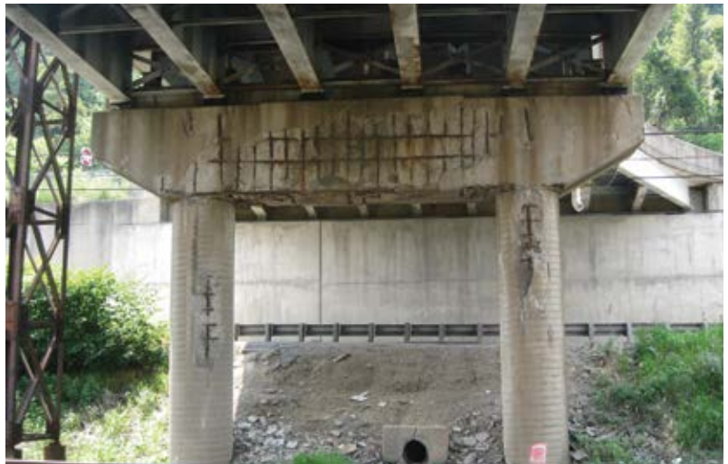
Fig. 3: This bridge pier scheduled for repair in the spring is adjacent to active rail traffic
