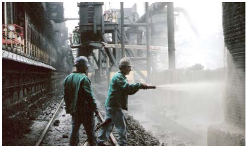
Fig. 4: During the shotcrete repairs to this coke plant quench tower, the railroad tracks are locked out with a derailer to prevent the use of the track while work is being done
