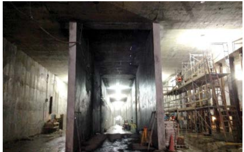
Fig. 4: Each of the three bays shown is a future train corridor for Long Island Railroad. To the right you can see square columns
