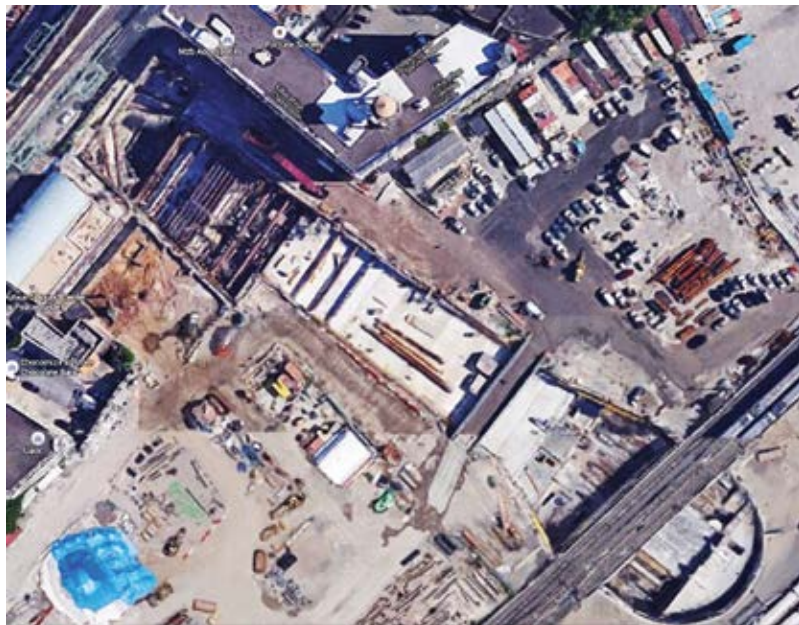
Fig. 1: CQ32 is a four-level ventilation facility, passenger station, and office for the MTA. Five other active projects are adjacent to and/or tie directly into the project, making logistics a challenge
