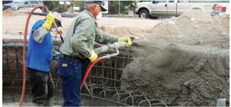
Fig. 5: ACI-certified nozzleman shooting walls with air-lance (blow pipe) tender cleaning the floor/wall joint before shotcreting so no rebound is used in the structure. Also, note the floor was completed first. The reinforcement at the bottom of the wall is for a bench that will be shot after the wall is complete. The contractor will need to clean all rebound and cuttings out from the bench area before shooting it
