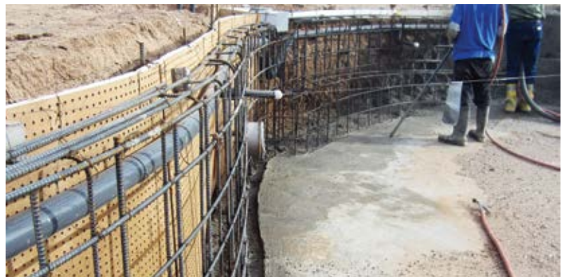
Fig. 7: Plumbing is a major component of most pools. Often, the plumbing components need to be placed in a way to allow for proper shotcrete placement. Enough room needs to be provided in the design for the plumbing, skimmer, lights, and reinforcing steel; pools take a lot of pre-planning with a qualified contractor and experienced crews
