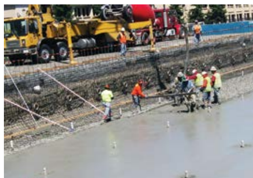
Fig. 3: Another pool floor being placed first with a concrete boom pump and the placement crew vibrating the concrete and screeding to the desired height. Installing the floor before the walls helps to guarantee no cuttings or rebound will be used in the structure. Also, note that a board is used at the edge of the floor to create a consistent joint. This allowed the joint to be prepped with water blast at 0.25 in. (6.35 mm) roughness before shotcreting the wall
