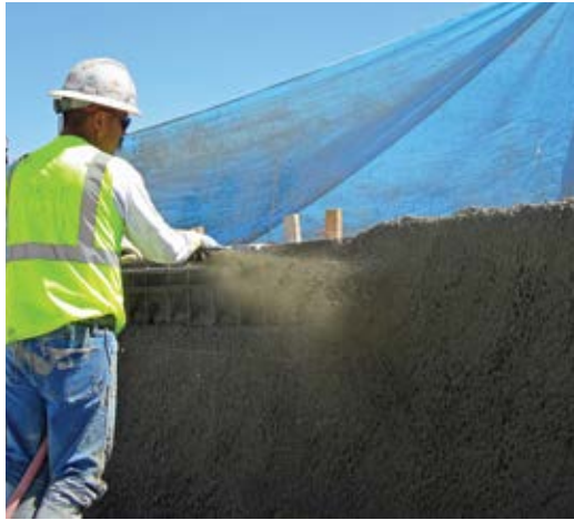
Fig. 4: Experienced ACI Certified Nozzleman shooting a beam—no cuttings will be reused in the structure. Also, note the blue tarp providing protection from overspray
