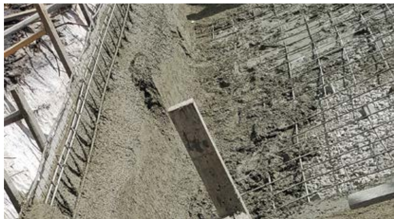
Fig. 1: A pool wall installed with wet-mix shotcrete before the pool floor has been placed. As a result, the pool floor is now contaminated with the rebound and cuttings from the shotcrete operation. This sloppy material sitting on the floor has not been vibrated or consolidated and must be considered as waste material and removed. Leaving this material in place would weaken the pool structure and significantly reduce the long-term durability of the pool shell. Unfortunately, incorporation of rebound and cuttings in the pool shell is the cause in 95% of swimming pool failures
