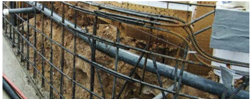
Fig. 6: When checking reinforcement, make sure the bars have proper clearance and cover. Reinforcing bars should be separated to meet the requirements of the project specifications and applicable local building codes. Stagger laps when possible to avoid bundling bars at contact laps, as seen at the top of the reinforcement in this image. Non-contact lap splices are preferred in shotcrete applications. Preconstruction shotcrete test panels may be required for contact laps that exceed No. 4 (No. 13M) reinforcement
