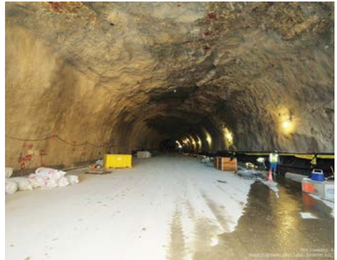
Fig. 12: Northbound view of the entire tunnel as seen from the south portal
