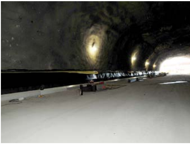
Fig. 9: Southbound view of tunnel after initial robotic placement of shotcrete for support
