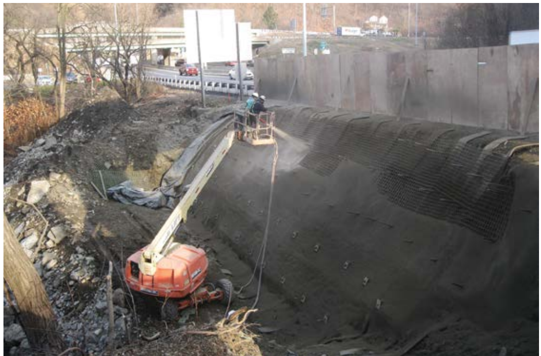
Fig. 1: Wooden barriers are installed in place along I-376 by the Fort Pitt Tunnel in Pittsburgh to protect traffic during the shotcrete placement of this soil nail wall
