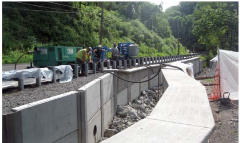
Fig. 4: On two-lane roads, when it is necessary to set up shotcrete operations on the roadway, a lane closure with advanced signing and flagmen becomes necessary
