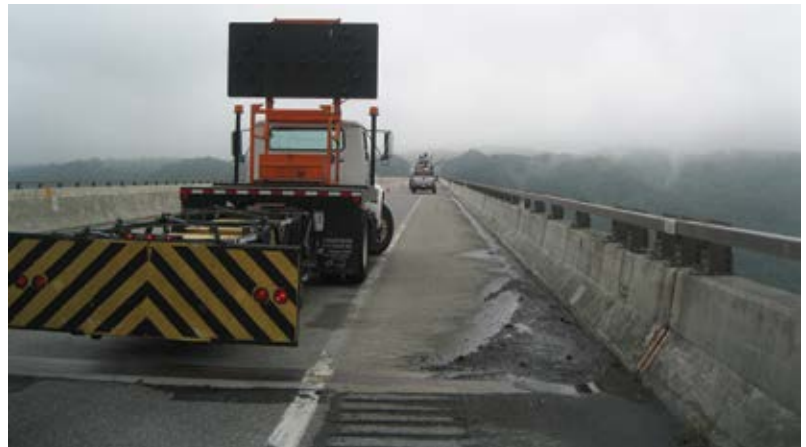
Fig. 3: Crash truck with impact attenuator and mounted arrow board, for a lane closure on a four-lane highway bridge in West Virginia
