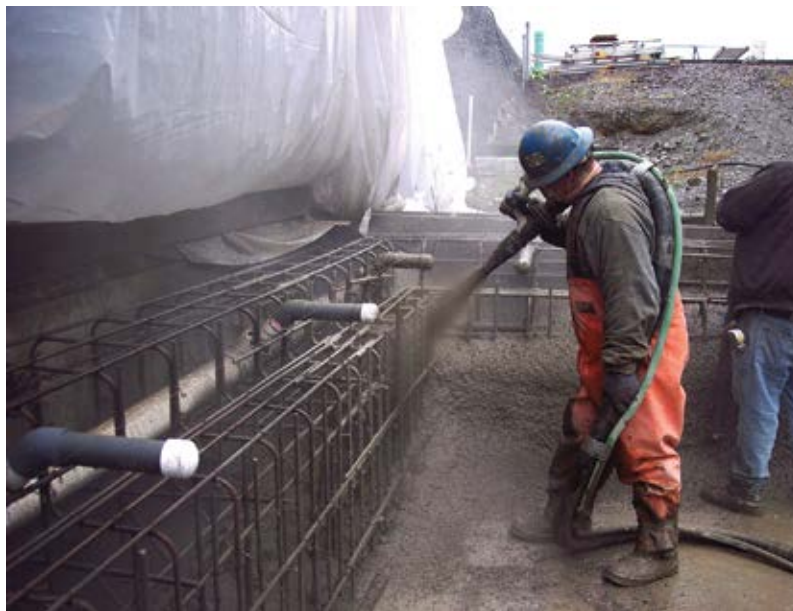
Fig. 3: Shotcrete sprayed at proper velocities results in compacted material with well-encapsulated steel reinforcing bar
