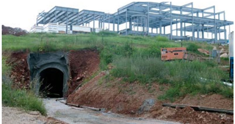
Fig. 3: Exterior portal leads to 150 ft (45 m) long tunnel and various chambers to create a wine cave 45 ft (14 m) under the owner's new home
