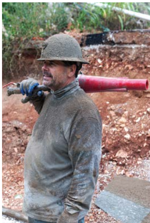
Fig. 1: Brady Mitchell is a modern-day cave man who specializes in wine cave construction, having built many in the Napa, CA, area
