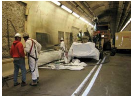
Fig. 2: Shotcrete being installed in the Liberty Tunnels by ACI Certified Nozzlemen using a predampener and a sufficiently sized air compressor. No damage to the tunnel was done by dust
