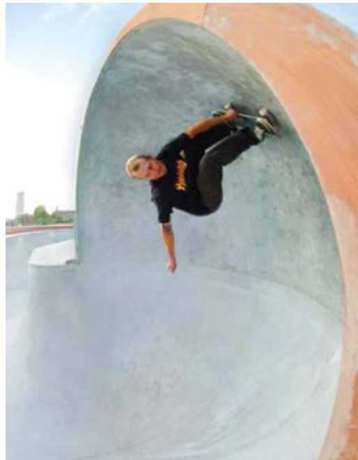
Fig. 3: Team Pain's Construction Superintendent, James Hedrick, testing the freshly placed "capsule" at the Kortrijk, Belgium, skatepark
