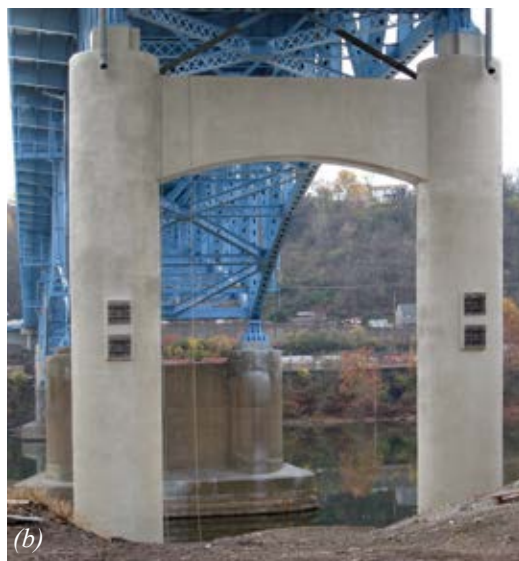
Fig. 1(a) and (b): Two large, round bridge piers being repaired and returned to their original contour using shotcrete
