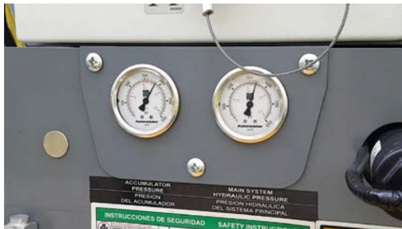
Fig. 5: Using hose only, this pump was pressuring out at 4600 psi (32 MPa) in the hydraulic system, or 1130 psi (7.8 MPa) on the concrete. Replacing 50 ft (15 m) of hose with pipeline lowered pressure to 3400 psi (23 MPa) in the hydraulics, or 835 psi (5.8 MPa) on the concrete
