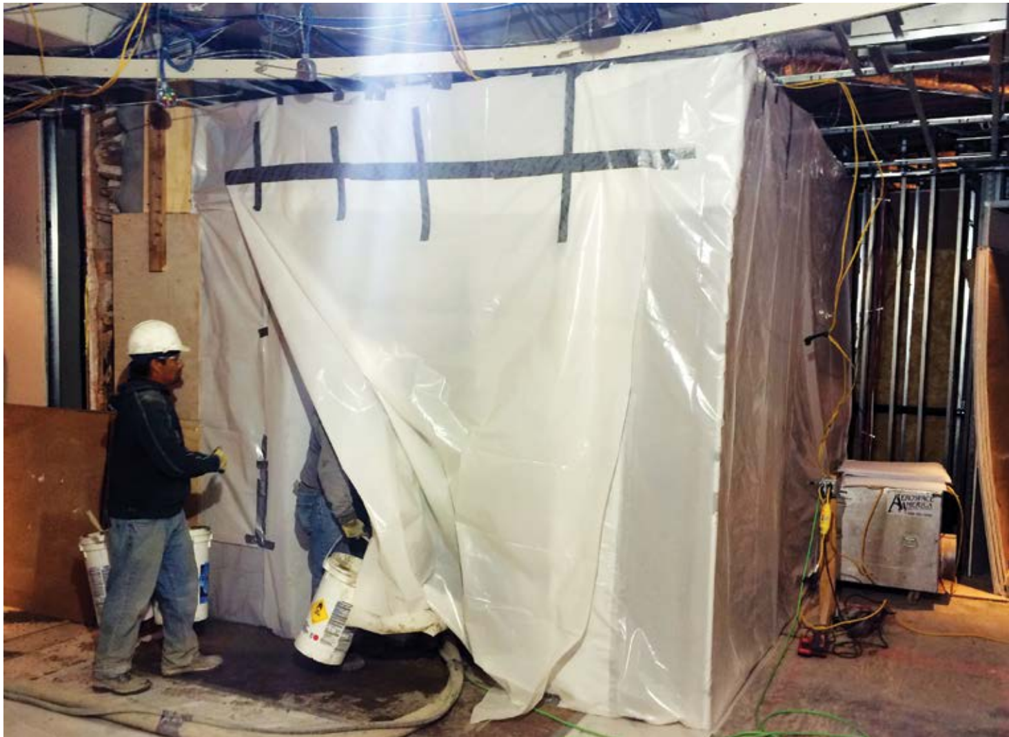
Fig. 1: This image shows an asbestos-like containment room to contain concrete repair work to its own area so that other trades could safely work around them
