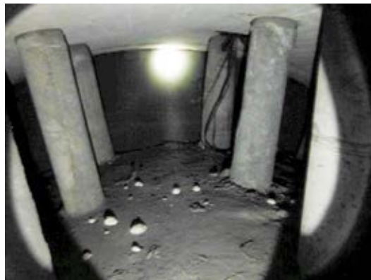
Fig. 6: Embedded hangers in existing void space between main tunnel and ventilation arch wall
