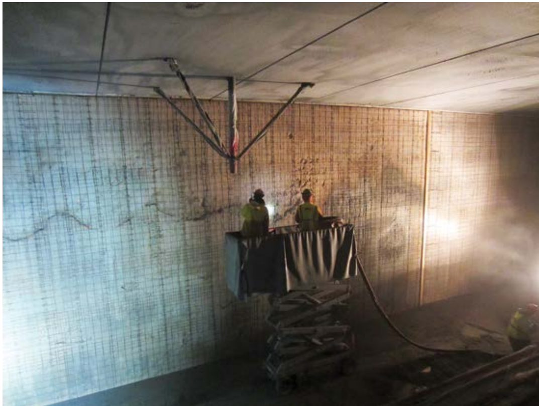
Fig. 3: Honeycomb at cold joint
