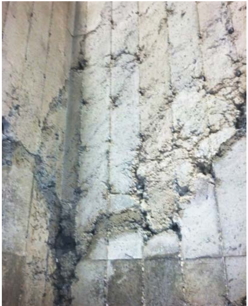
Fig. 2: Poorly consolidated concrete
