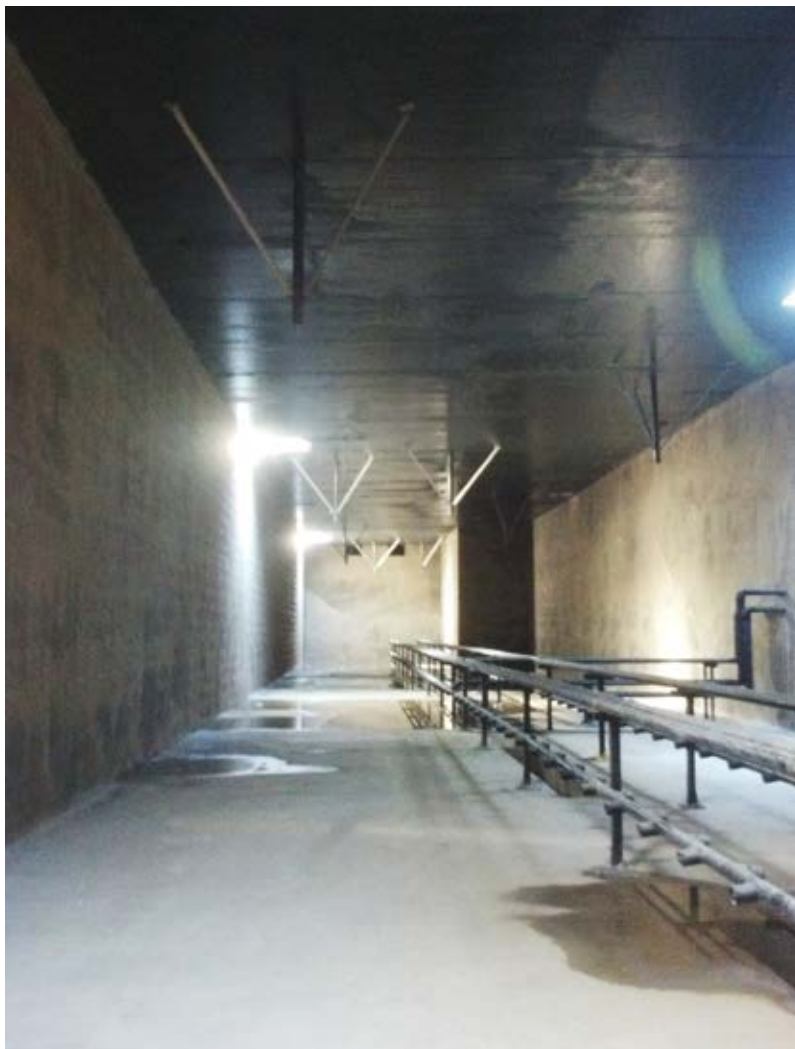
Fig. 1: Tank before repair
