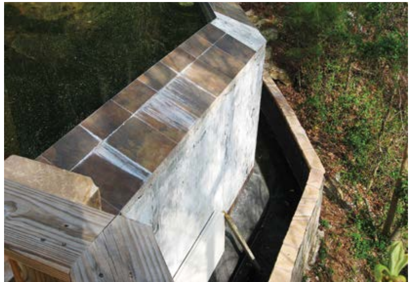
Fig. 4: Efflorescence buildup that caused delamination of tiles; more than just an aesthetic problem
