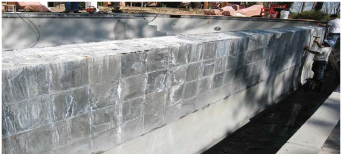
Fig. 1: Infinity edge (water-retaining wall) of swimming pool—2-year-old pool with no specific integral waterproofing or densifier controls
