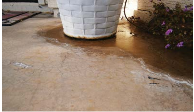
Fig. 3: Aged concrete slab deterioration
