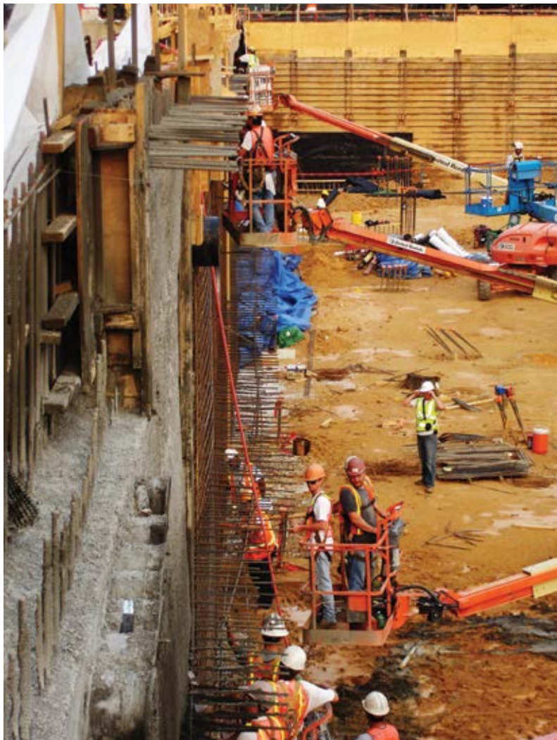
Fig. 1: Lagging and steel I-beam piles with soil anchors. Waterproofing installers and reinforcing bar crew working just ahead of the shotcrete crew
