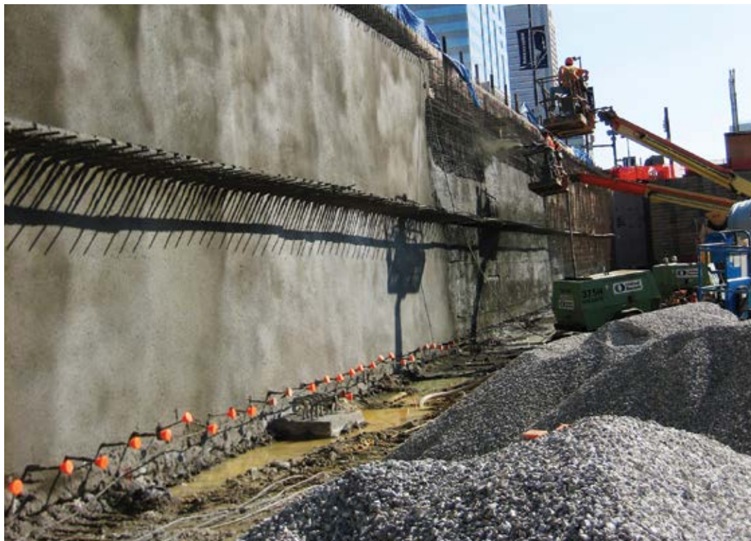
Fig. 10: Finished wall with other trades stockpiling gravel for the floor installation following right behind
