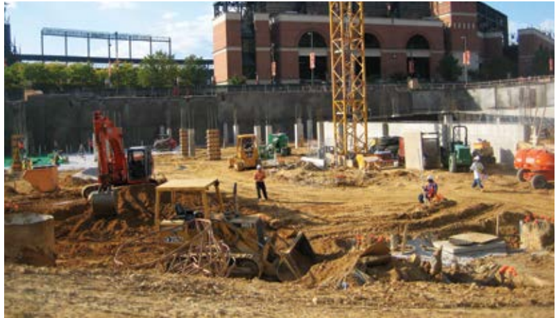
Fig. 6: Different operations on this project were trying to get in and work making it difficult to perform the shotcrete placement while staying out of everyone's way
