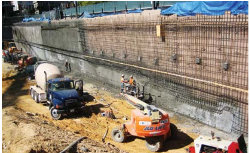
Fig. 7: Keeping the walls and reinforcing steel wet in front of the shotcrete was a challenge so as not to activate the bentonite waterproofing or create a muddy mess for the equipment to drive on
