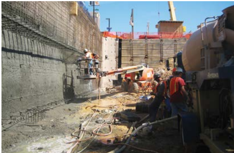
Fig. 8: Tight working conditions Coastal had to work in daily to allow other trades to work. The wall waterproofing and reinforcing bar installation had to stop due to the dirt ramp that was in the way. Spraying water on the walls made a muddy mess and had to be dug out, replaced, and compacted before any equipment could be driven over it
