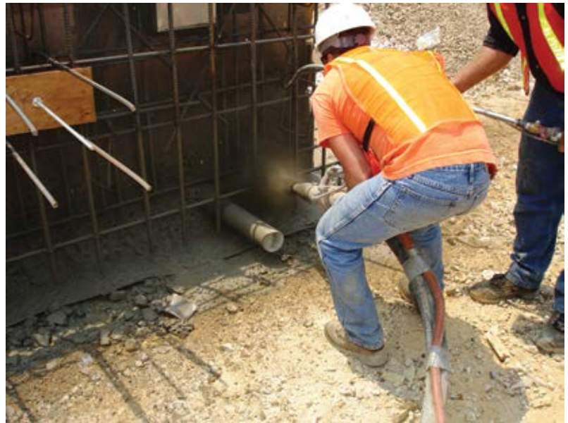
Fig. 3: Mockup with waterproofing—one of many reinforcing bar and waterproofing configurations Coastal faced. The blowpipe operation was key to keeping the rebound, overspray, and water out of the wall sections
