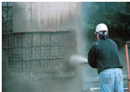
The dry process of shotcrete being gunned on a pier can provide a better bond without using bonding compounds. The nozzleman is filling in the corners first and working toward the middle of the repair area so he doesn't trap rebound in the corners
