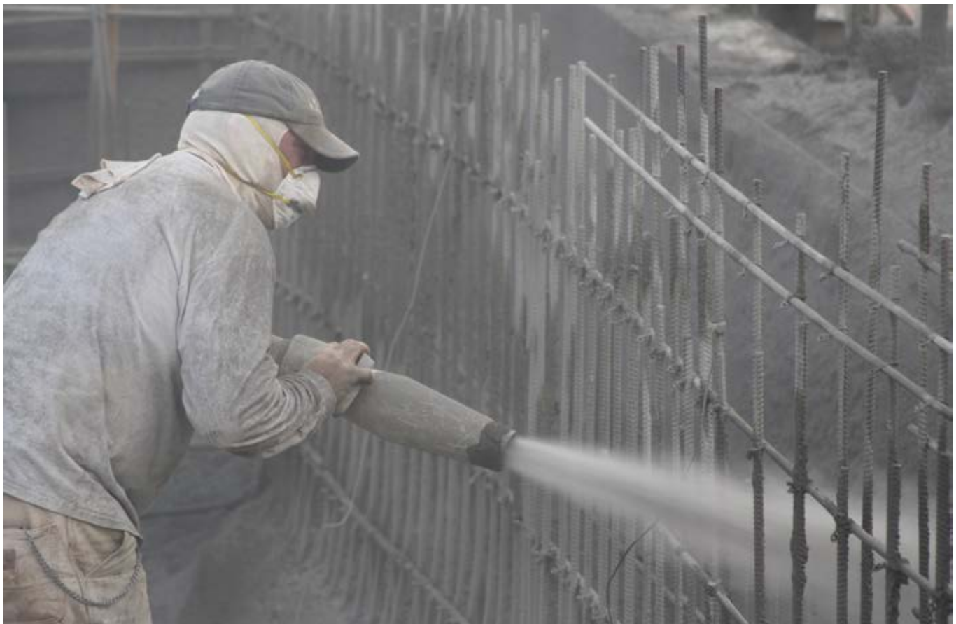
Fig. 1: Dry-mix shotcrete being applied to catch basin wall from inside of the pool due to space in catch basin (Willie Johnson, NP Superintendent, ACI Certified Nozzlemaster)
