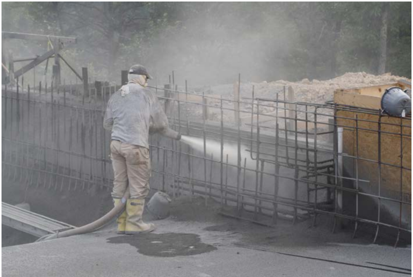
Fig. 2: Shotcreting the exterior wall of the vanishing edge catch basin before edge wall is formed and shot
