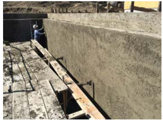
Fig. 4: The final layer shot and cut, waiting to receive steel trowel finish
