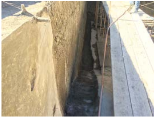
Fig. 2: First layer is ready to receive its final layer once SSD is achieved
