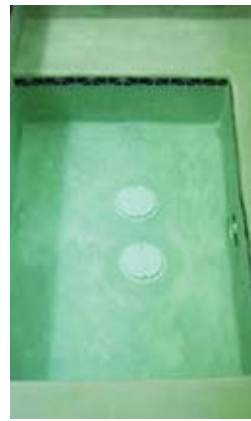
Fig. 5: Hydration issue due to variation in plaster thickness at dig outs
