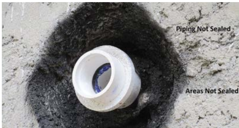
Fig. 4: Improper sealing at pipe-shotcrete transition, leaving unsealed areas. Applying a sealant to the entire dig out area that is not compatible with cementitious materials
