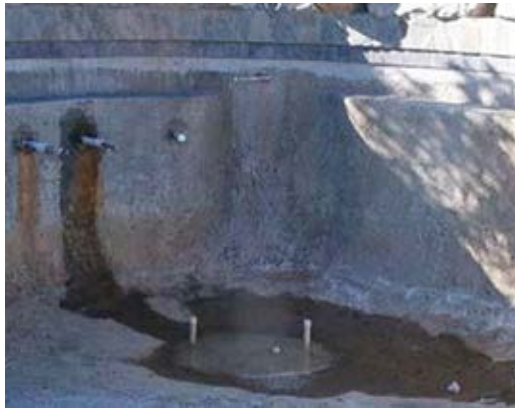
Fig. 1: Water intrusion at penetrations from behind structure
