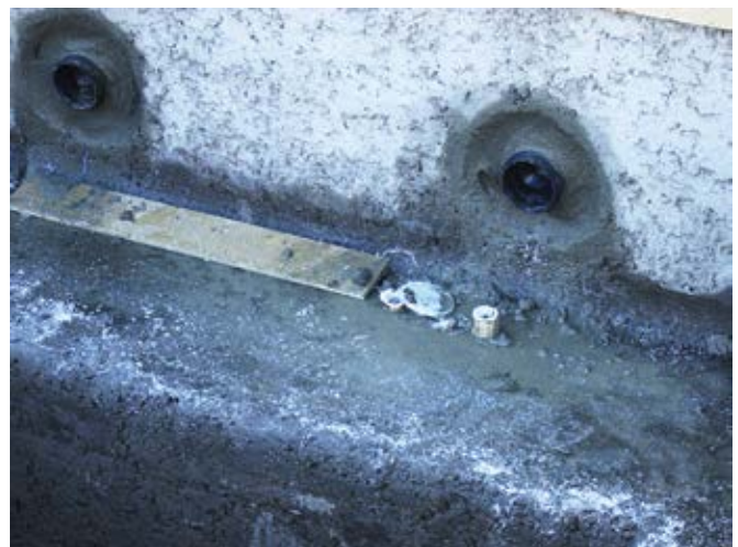
Fig. 3: Piping with fittings and sealed
