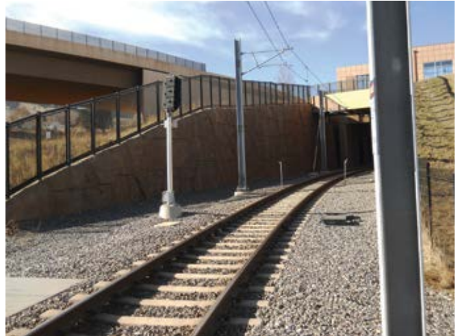
Fig. 2(b): Light rail station east section retaining wall showing support for adjacent bridge abutment
