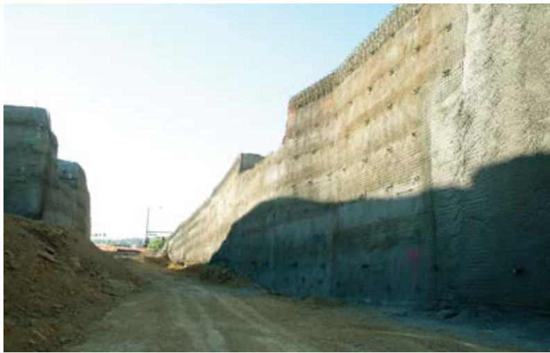
Fig. 1(a): Jefferson County Government station under construction. Full depth—33 feet (10 m)—supporting adjacent highway with permanent soil nails and shotcrete (Photo courtesy of Harry Olsson)
