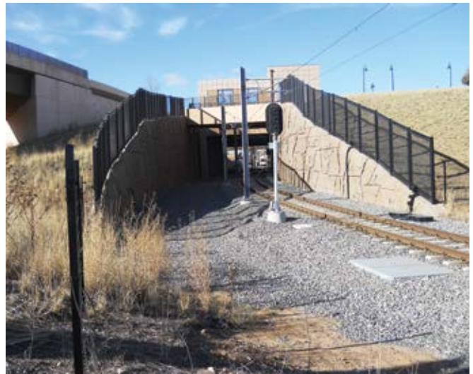
Fig. 2(c): Light rail station showing shotcrete and soil nail support for tunnel out of station
