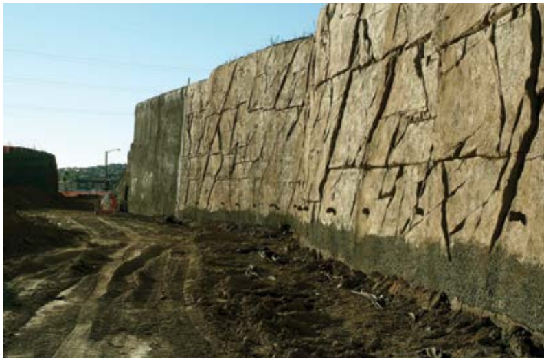
Fig. 1(b): Wall under construction showing carved shotcrete facing, which is also structural member of final permanent wall structure (Photo courtesy of Harry Olsson)
