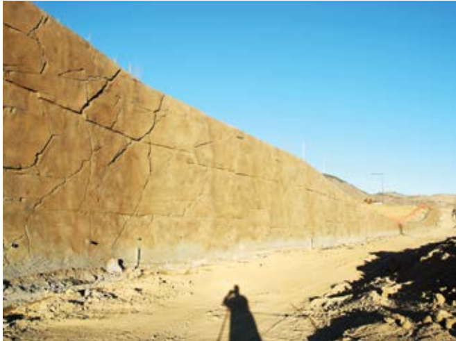
Fig. 1(c): Extent of shotcrete station wall before backfill of drainage and rail bedding (Photo courtesy of Harry Olsson)
