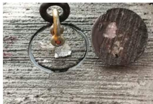
Fig. 5(a): Picture of glue plane failure
