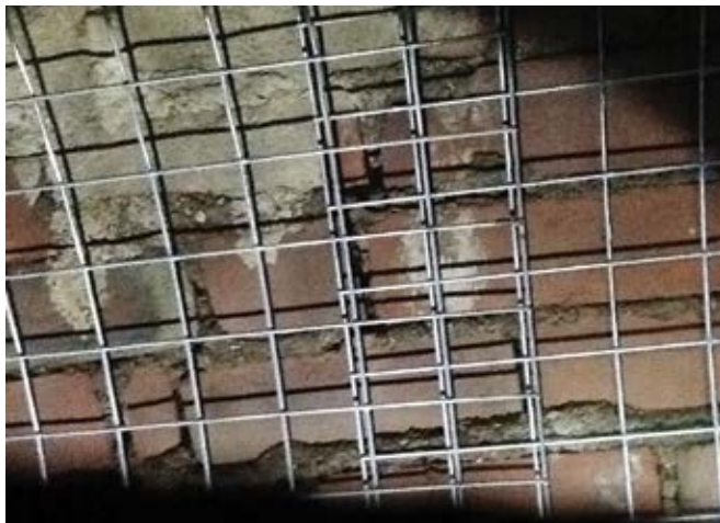
Fig. 3: Close-up of wire reinforcement lap and brick substrate
