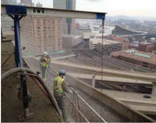
Fig. 2: Due to restricted access and nothing above to suspend cables from, outriggers were used to hang swing stages for the shotcrete rehabilitation work
