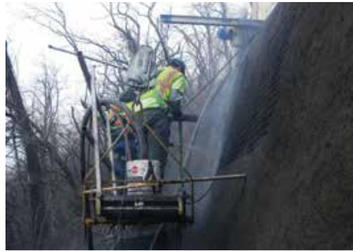
Fig 5: Nozzleman and cutdown man working together to complete upper areas of the eastern wall
