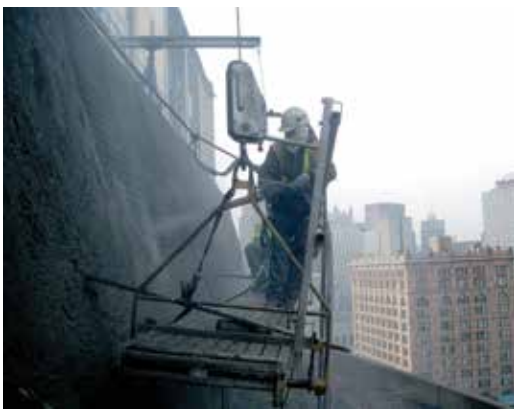
Fig. 4: Nozzleman on suspended swing stage, turning to his side, to get enough distance from the wall to get a good spray pattern
