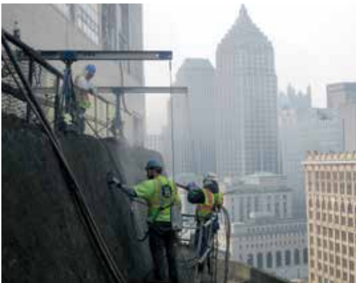
Fig. 3: Shotcrete is placed with Pittsburgh landmarks the Gulf Tower and Koppers Building in the background
