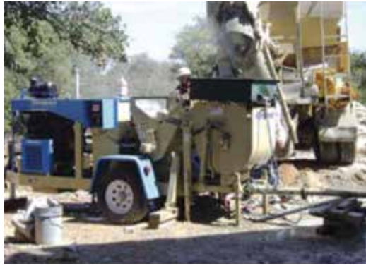
Fig. 12: An Allentown Powercreter 20 is shown with a hydraulic mixer attachment. The attachment is being used as a remixer for concrete supplied by a mobile, or a volumetric mixer for site batching to achieve a consistent mixture for pumping operations. A vibrating screen was installed to reduce the risk of plugging the 1.5 in. (38 mm) hose due to randomly occurring large aggregate particles. The electronic control technology produced a continuous flow of concrete material that allowed the nozzleman to apply a uniform shotcrete layer to the walls with very little line surge. The unit can pump concrete containing up to 1 in. (25 mm) stone mixes through a 4 in. (100 mm) hose
