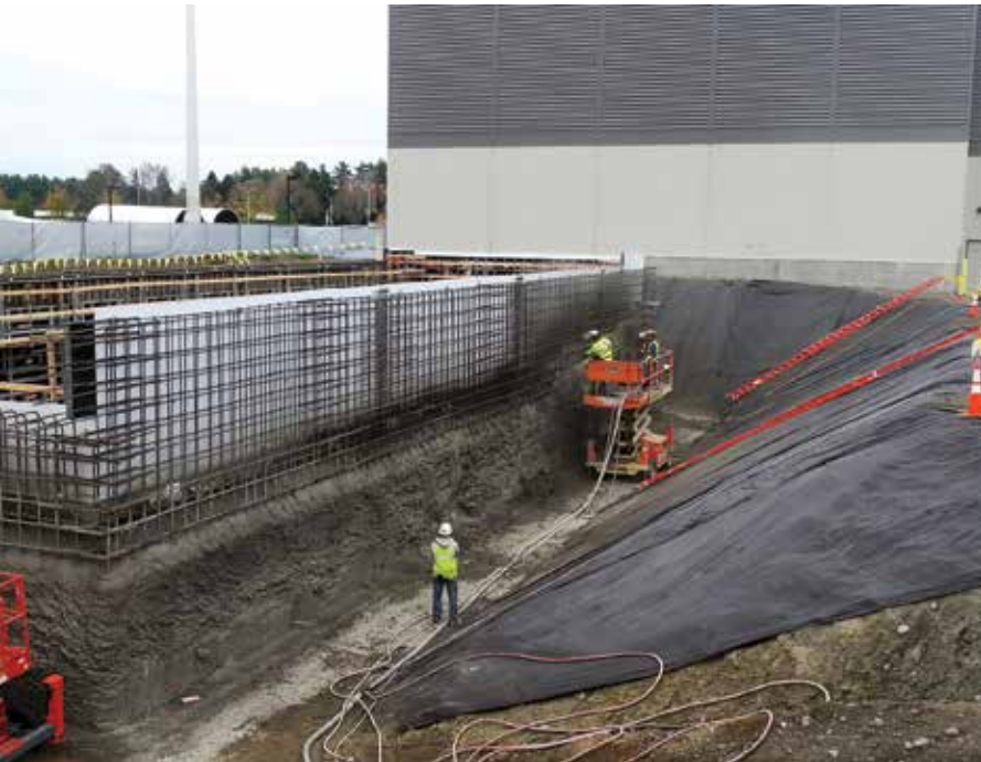
Fig. 2: Nozzlemen using scissor lift instead of scaffolding to gain access to the 270 ft (82.3 m) perimeter research tank project
