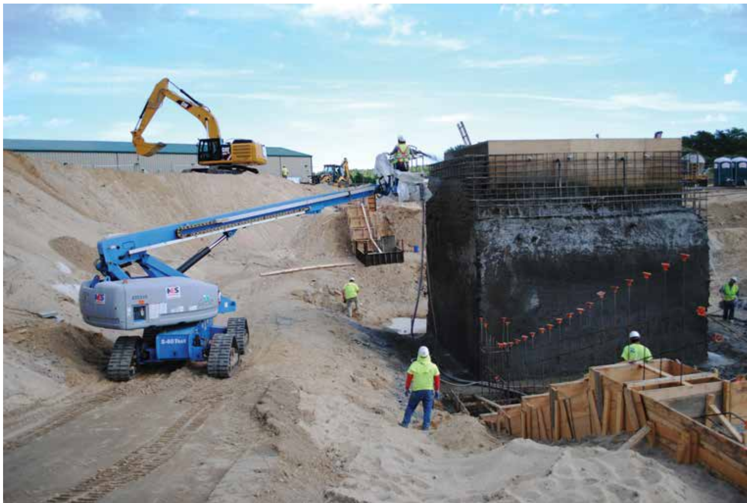
Fig. 1: Nozzlemen shooting a research tank from a lift. The site had terrible soil, which required an all-terrain lift with tracks instead of wheels to give safe access for nozzling and finishing
