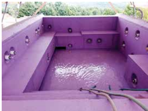
Fig. 1: A spa with a purple-colored waterproof membrane, undergoing a flood test prior to tile installation
