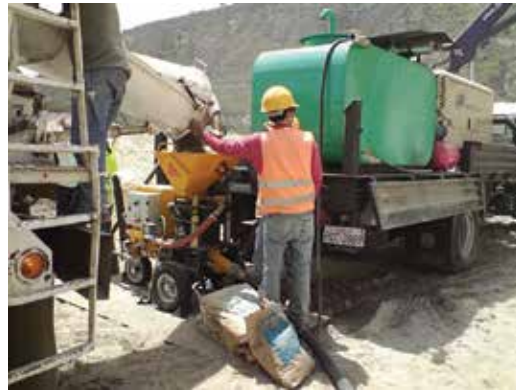
Fig. 2: Slope stabilization with Aliva-257 in Quito, Ecuador. One of the new roads leading to the new airport
