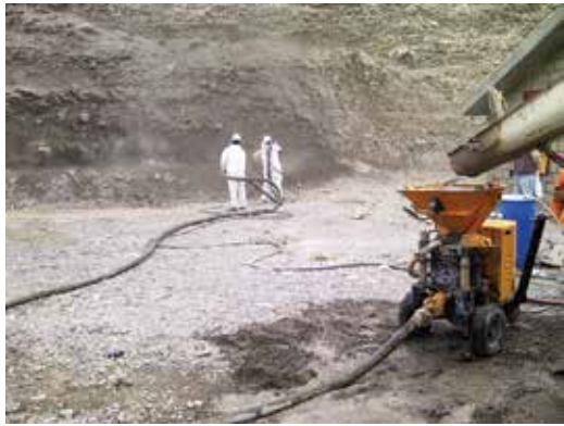
Fig. 1: Practicing slope stabilization with wet concrete in Arequipa, Perú, with an Aliva-257
