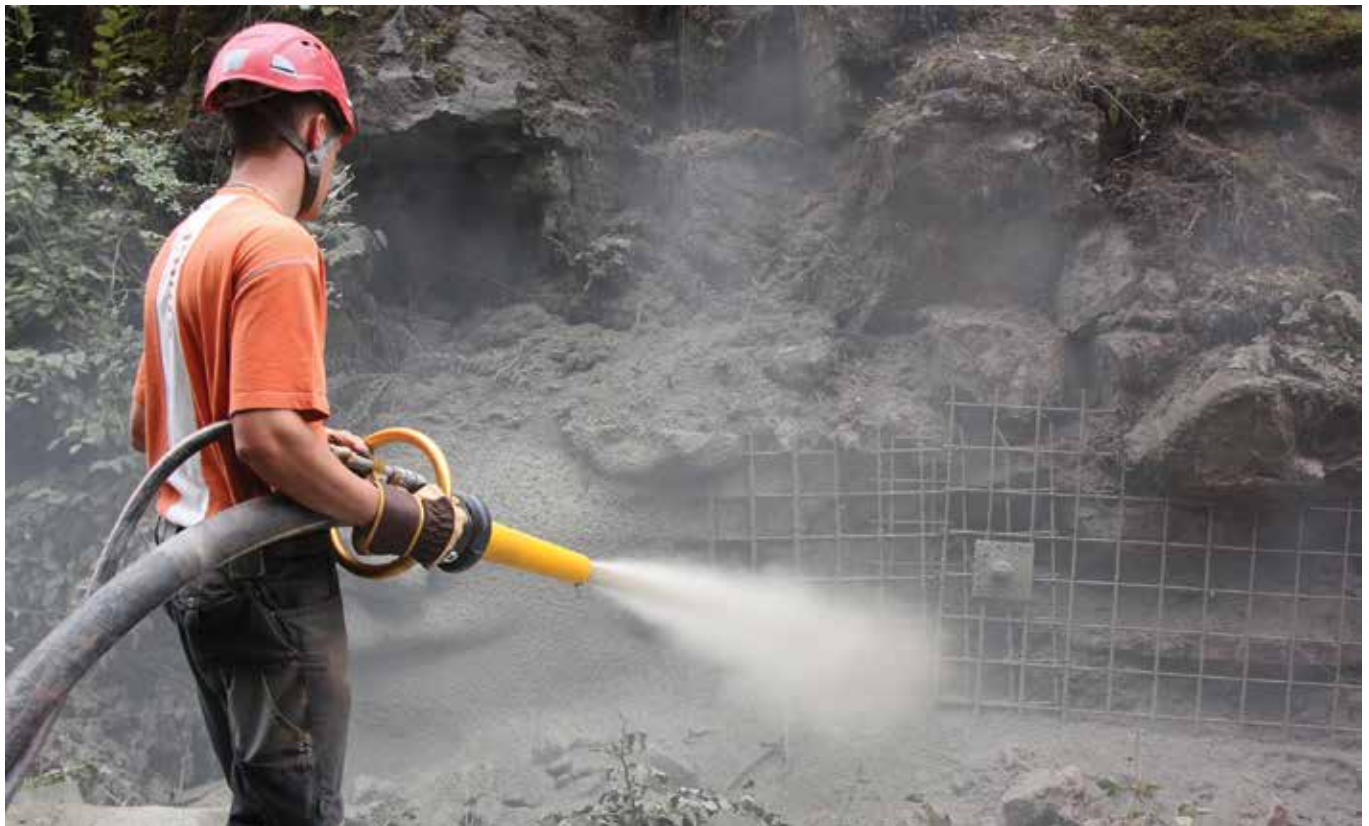
Fig. 3: Stabilizing rocks with wet concrete with Aliva-257. Here, the new Converto manual spraying gun is used
