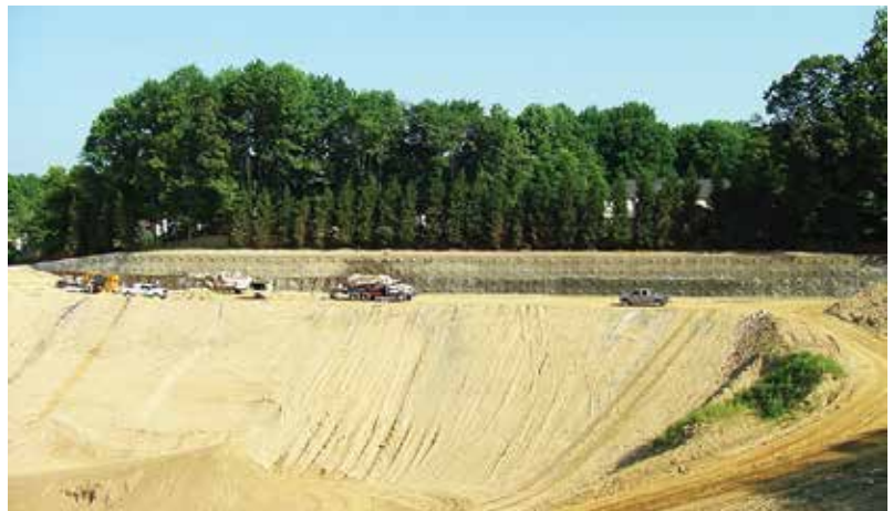
Fig. 4: Access roads were built and drilling commenced, closely followed by nail grouting and wire mesh installation
