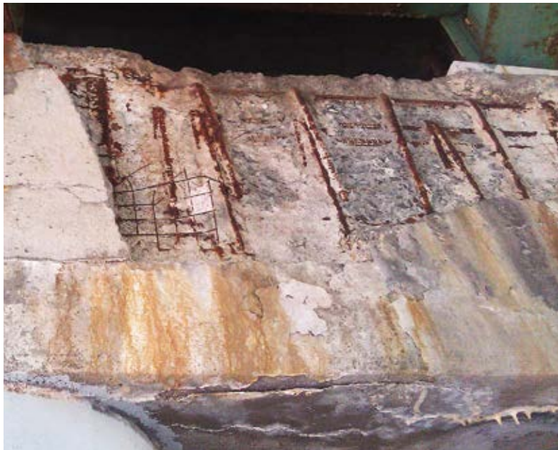
Fig. 1: Corrosion damage on concrete bridge pier
