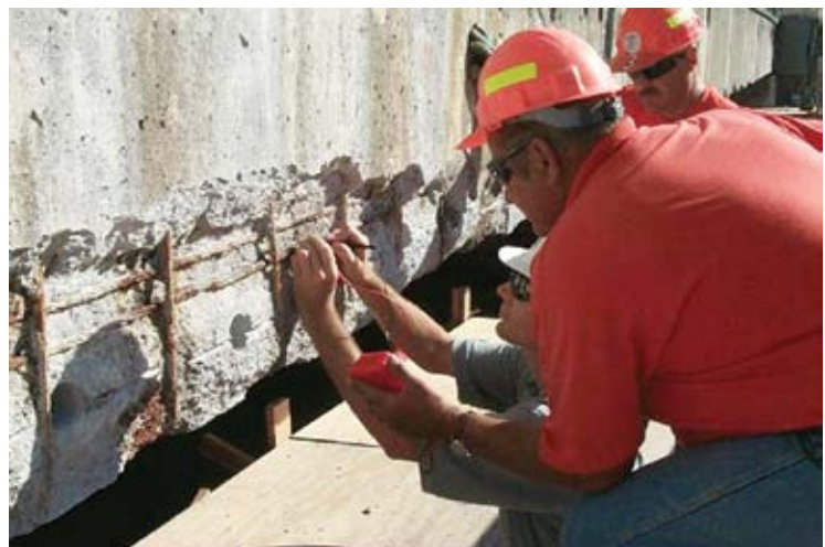
Fig. 6: Type 2 anodes placed into holes drilled into the parent concrete and connected to the steel in the repair
