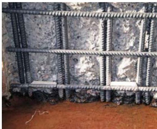
Fig. 10: Thin elongated anodes installed prior to shotcrete repair. Installation behind the reinforcing bar further reduces cross-sectional area
