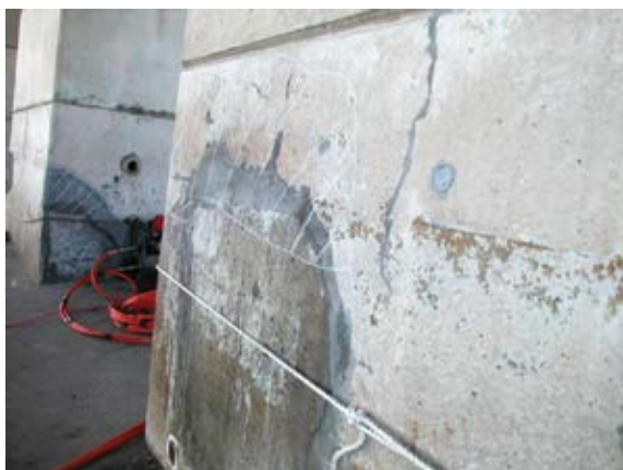
Fig. 2: Patch-accelerated corrosion in parent concrete around previous repair
