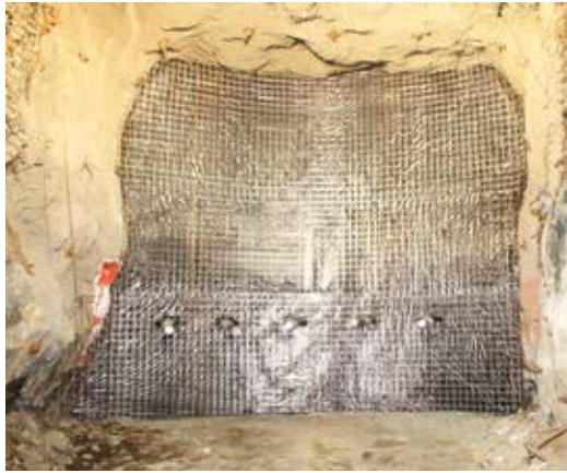
Fig. 1: Construction of original shotcrete backfill barricades involved the use of panels constructed using two layers of welded wire reinforcement, separated with spacers to act as a vehicle for the shotcrete. Fabrene was usually fastened to the back of the first layer of mesh to provide a receiving surface for the shotcrete
