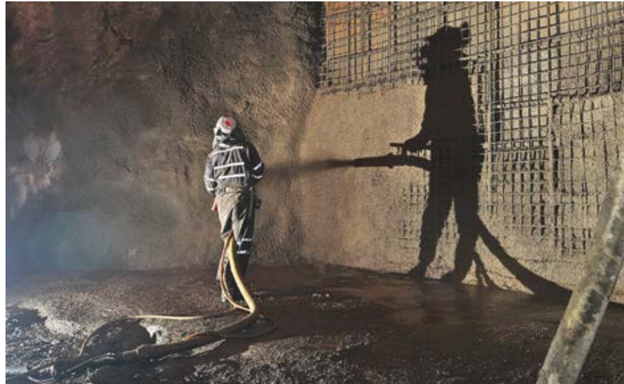
Fig. 2: Reduced manpower, reduced cycle time, and improved water retention soon made the shotcrete process the preferred method for constructing backfill barricades
