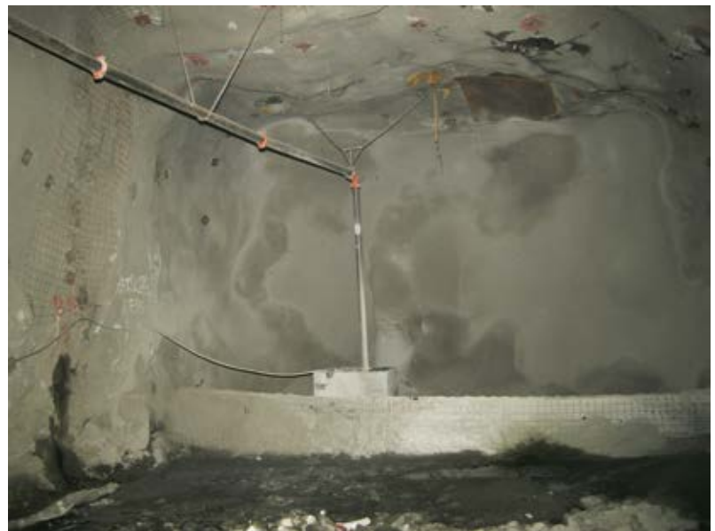
Fig. 3: A completed backfill barricade in a northern Ontario mine was constructed using the shotcrete process (note drainage pipes that allow water to drain from the backfill material)
